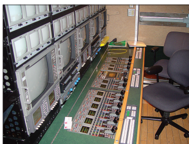
Figure 3.54 Video compartment of a truck under construction. Each large black knob represents iris and black level control of a camera. The panel between the controls for the eighth and ninth cameras allows for more detailed control and setup of any of the cameras.
