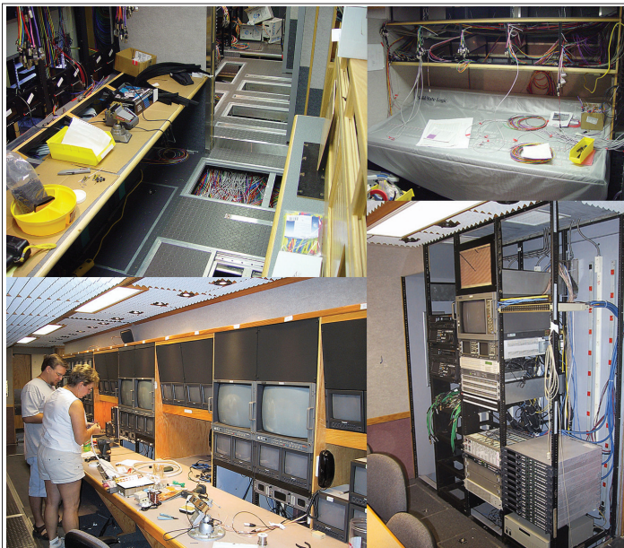
Figure 3.53 Equipment is installed and wired into a complete system. (Source: Core Digital Technologies/SWTV and Bennett Systems)
